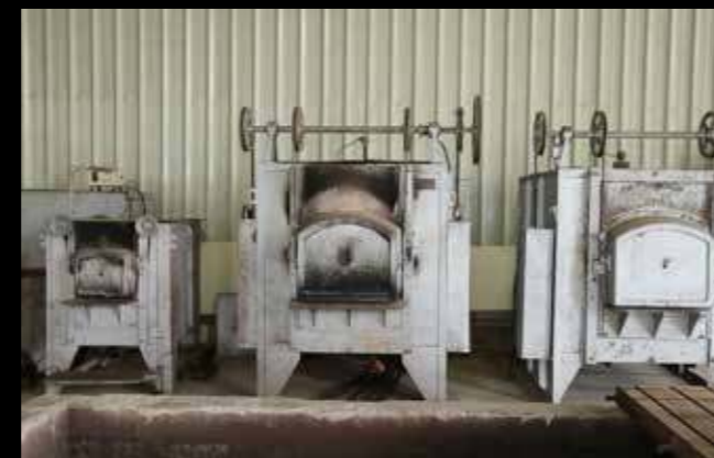
Chamber furnace system for heat treatment
