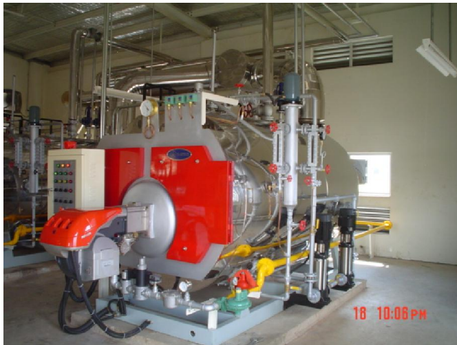
Picture of a boiler using diesel fuel.
